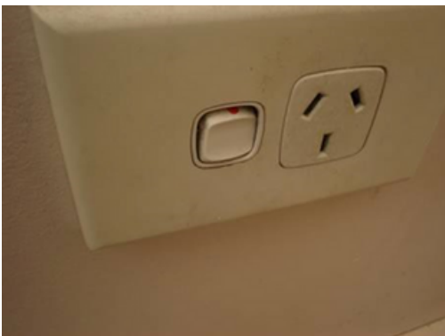
A loose switch to a power point needs repair as soon as possible
