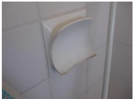
This broken soap dish in the shower could cause injury and needs to be replaced.
