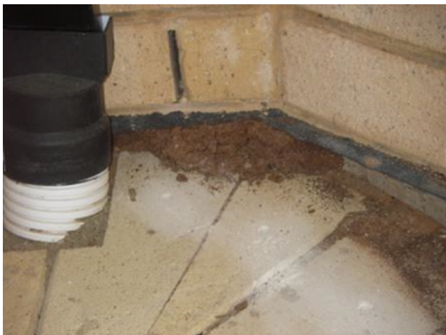
These mud deposits indicate active termites
